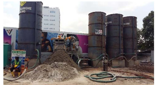
Desanding and Benonite Silos
