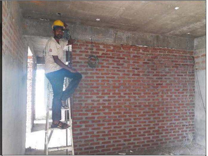
Figure 3.8 – 3 rd floor soffit wiring
