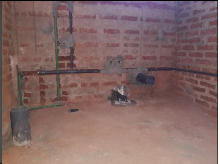
Figure 3.8 – 2 nd floor bathroom plumbing
