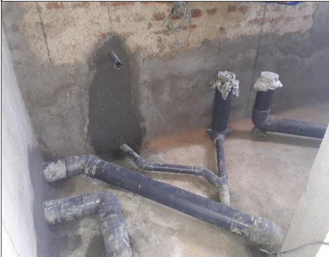
Figure 3.9- 2 nd floor bathroom plumbing
