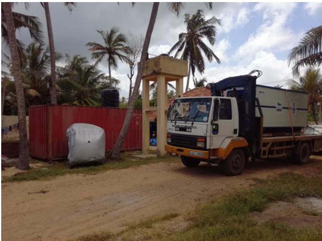
New generator bought to speed up work
