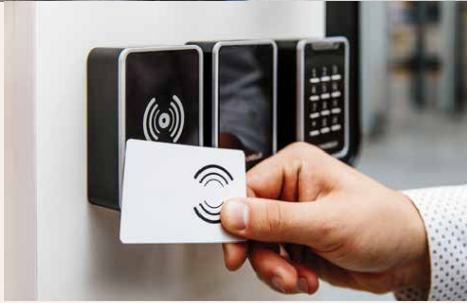
ACCESS CONTROLLED ENTRY
